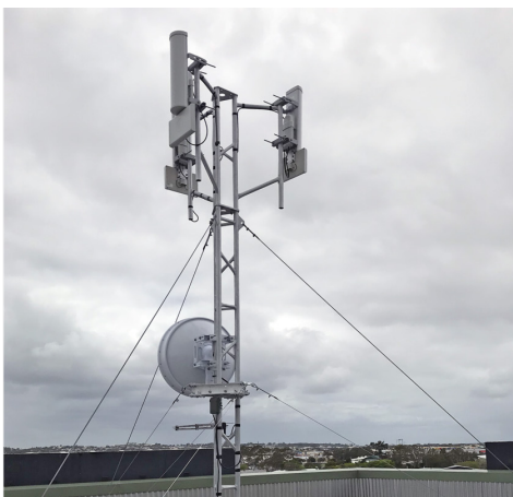
Figure 12: Sector Wi-Fi Tower with Point to Point Radio on the bottom. (Source: Blackhawk Antennas)
